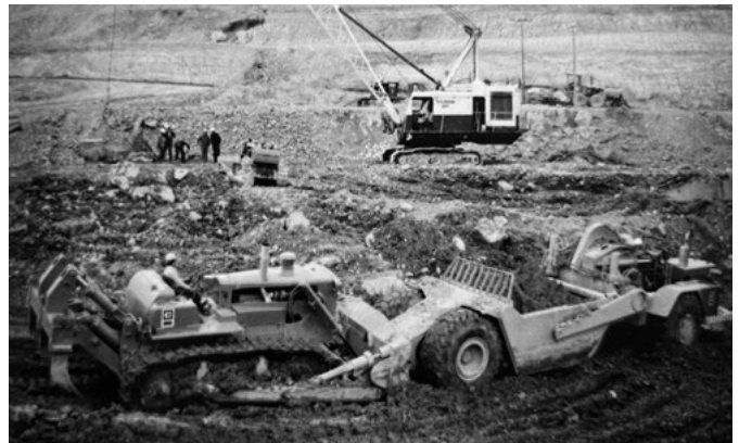
Removal of pug material from downstream of the original Pukaki Dam site before construction could start on the new intake and spillway structures of the new Pukaki High Dam. In the background is a Marion 111 crane rigged as a drag line.
