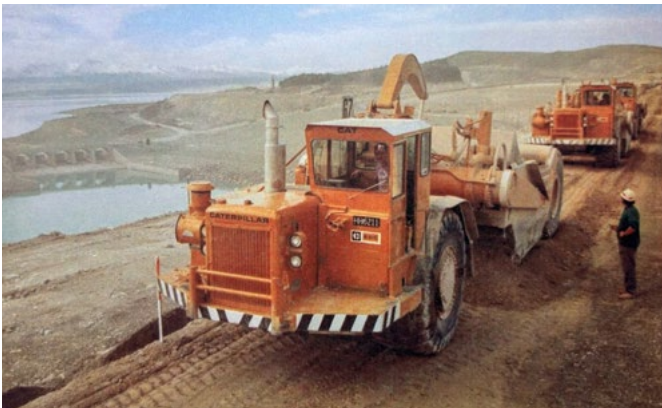
G&M Caterpillar 631C scraper fleet number G7 followed by two more 631C scrapers lay the final layers of fill into the dam core. Below the high dam can be clearly seen the old Pukaki dam which was flooded to raise the lake to its present level.
